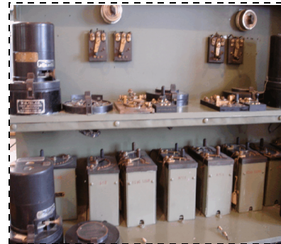
Repeaters at Hearts Content convert cable signals to land line circuits
